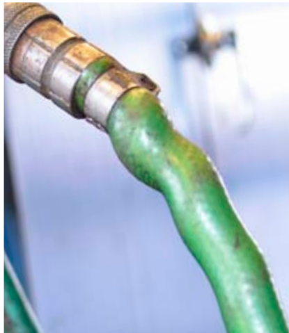
Old coupling with hose clamps causing leakage and pressure drop
