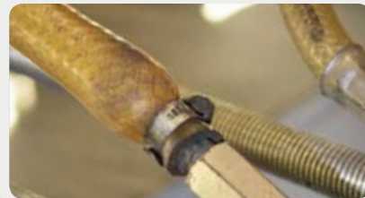
An illustrative example of a leaking coupling with hose clamp.
